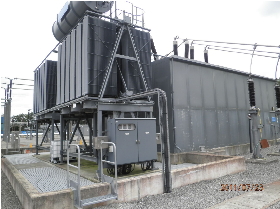
Figure 4.3: Typical (large 400kV) Power Transformer
